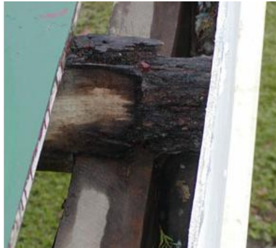
Deteriorated timber (Floor joist at external wall connection)
