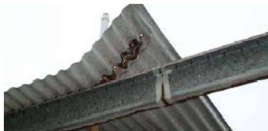
Corroded screws and cladding
