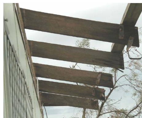
Corroded batten straps
