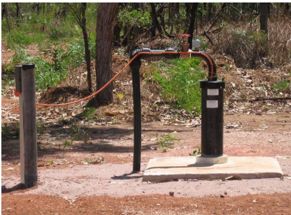
Photo 2 - AN EXAMPLE OF A BORE THAT HAS BEEN CONSTRUCTED AND EQUIPPED TO STANDARD
