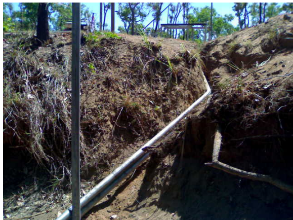
Photo 7 Example of Orifice line / Gal Pipe
