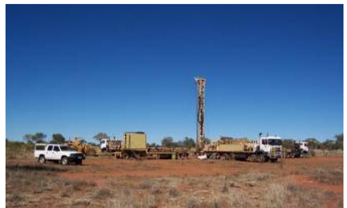
A NT Government drilling team constructing a monitoring bore in the Ti Tree Water Control District
