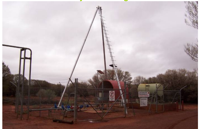
Photo 2 – Satisfactory Fuel Storage
