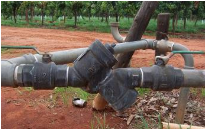
Picture: (below) A much smaller (50mm) RPZD that is utilised to protect not only the resource but also preventing cross connection with the shared domestic supply.
