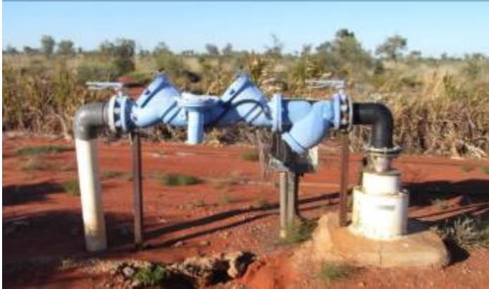
Picture: (above) a 150mm Reduced Pressure Zone Device (RPZD) – Suitable for situations in which there is a high hazard level. This example being a major agricultural property that utilises chemical and fertiliser injection into the irrigation lines.
