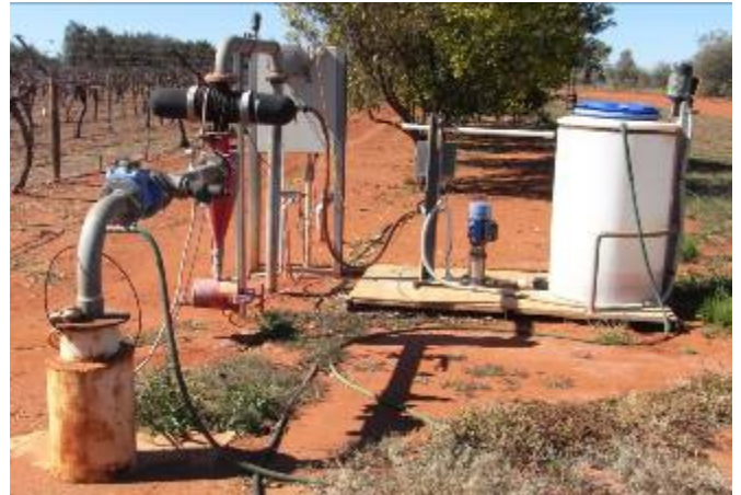
Picture: High risk of contamination through Backflow (i.e. back-syphoning) with the hose used to fill the chemical or fertiliser mixing reservoir is left in place unattended, with no backflow prevention device apart from a manual shut-off valve.
