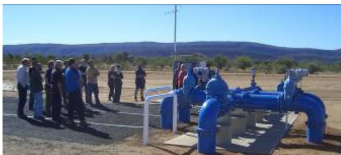
Remote-controlled pumps, pipes and valves distribute treated water evenly into the infiltration basins for underground aquifer storage and later recovery and use
