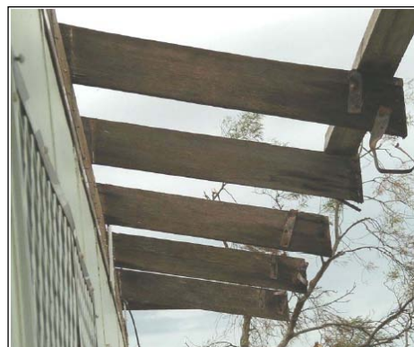
Corroded batten straps
