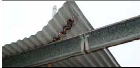
Corroded screws and cladding
