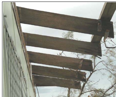
Corroded batten straps
