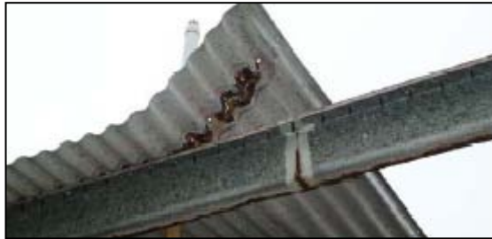
Corroded screws and cladding
