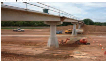
Below: The Cycle Bridge with all beams and precast elements in place.
