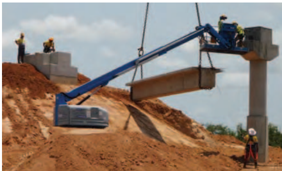
Above: The first beam in the cycle bridge is lowered in to place in December 2009.
