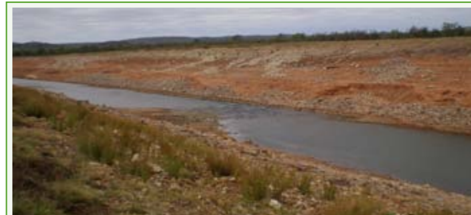
Minor slumping erosion and scour can be seen along the McArthur River diversion channel. Vegetation establishment, may help stabilise the banks of the diversion throughout the wet season floods. (May 2010)
