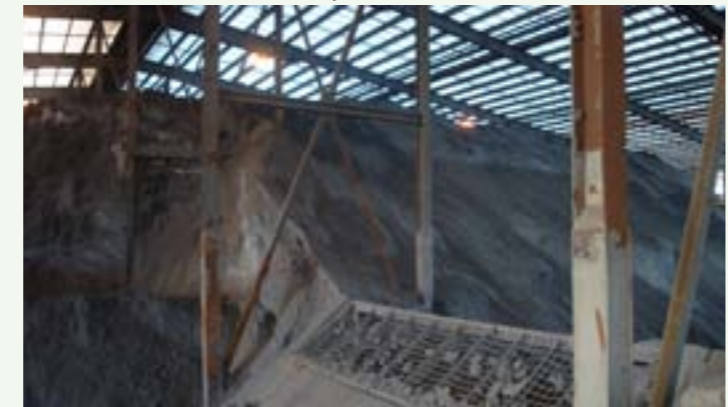
Zinc concentrate is stored within the Bing Bong concentrate storage shed while awaiting loadout onto the Arburri barge for shipment. The doors of the shed remain open to limit gas build-up that corrodes shed infrastructure. However, the open doors also allow concentrate dust to escape and spread via the wind to potentially contaminate soil, water or and sea sediments. This past year, damaged sections of the warehouse corrugated iron roof were replaced with fibreglass roofing that is resistant to the corrosive gases. The upgrade of the roof will assist in reducing dust emissions at the load out facility
