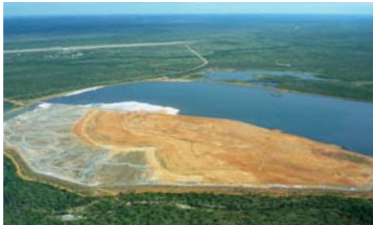
The clay capping of TSF Cell 1 was approximately 60% complete during our inspection in May 2010, as seen above. The rest of the capping is to be completed by the 2010/2011 wet season to reduce infiltration of water through the exposed tailings and reduce dust generation.
